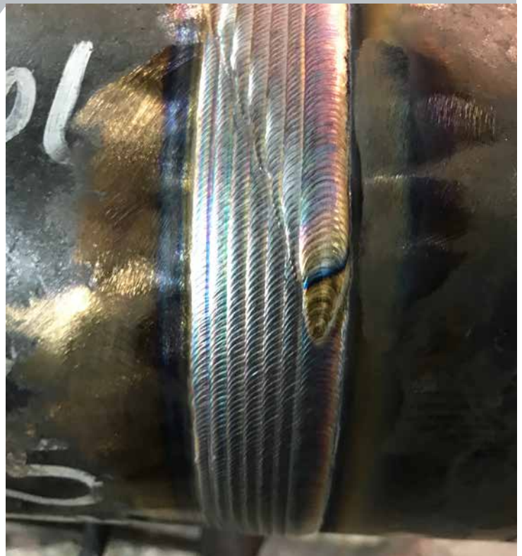
In the photo above the TIG process was utilized from the root pass continually through the cap passes on P91. Tri Tool AdaptARC equipment delivers reliable high-deposition rates.
