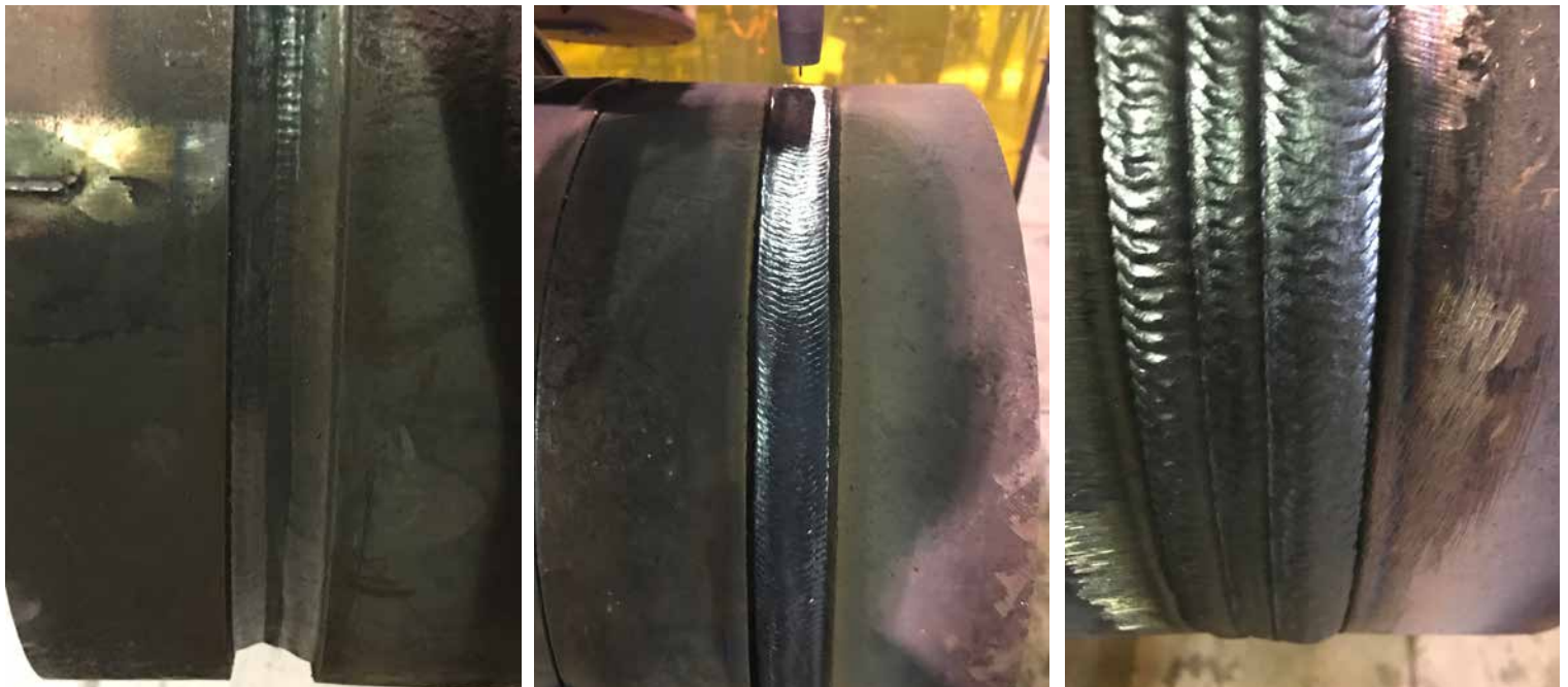
A sequence of photographs (from left to right) showing a weld procedure development involving using automatic fluxcore 1/16" welding wire on carbon piping. After completing and demonstrating weld development on the mock up, the above process was then successfully implemented at a nuclear plant, being used for a 32" FAC pipe replacement project.
